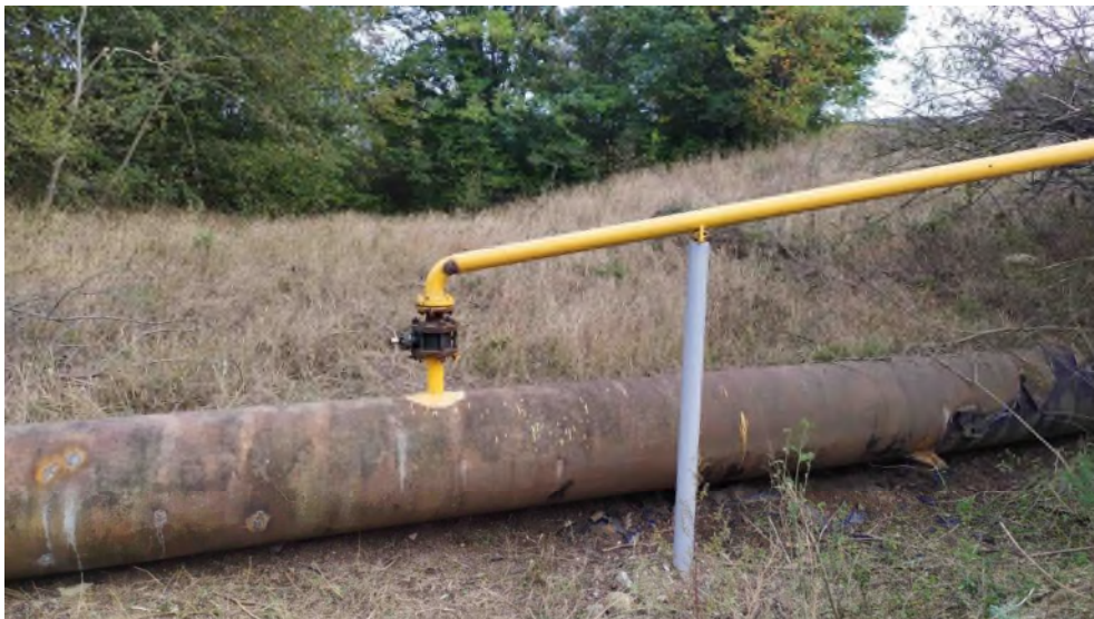
Figure 20. The Main Gas Pipeline in Stepanakert City Struck by Azerbaijan
