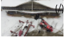
A collapse occurred on the roof of the bus station, where excessive snow accumulated (/video/amasyanin-tasova-ilcesinde-asiri-kar-biriken-otogarin-catisinda-cokme-olustu-1903056?utm_medium=Video%20Haberler%20Widget&utm_source=Cumhuriyet&utm_campaign=Video%20Haberler%20Widget)
